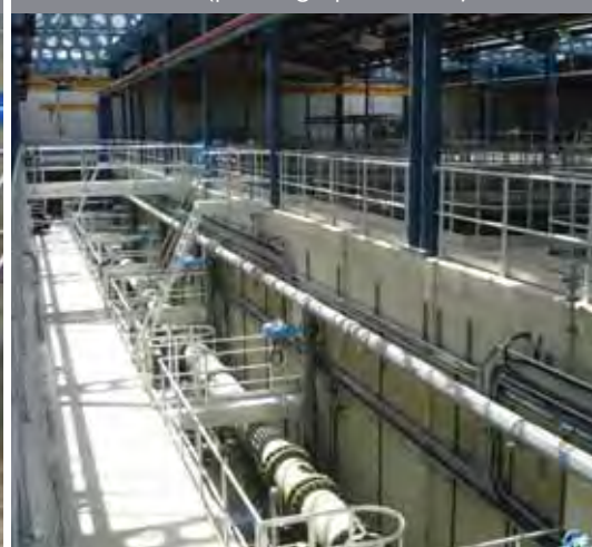
Headingly Water Treatment Works
