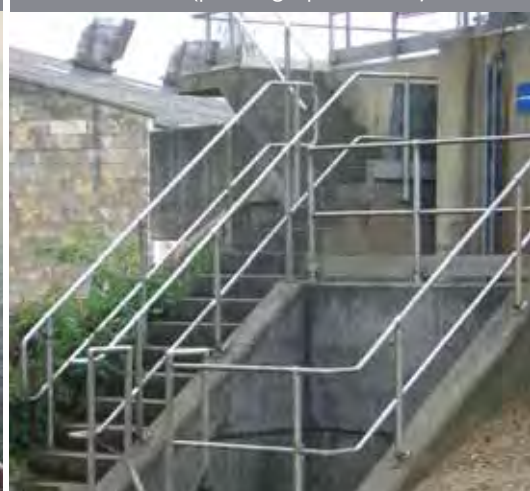
Tadcaster Water Treatment Works
